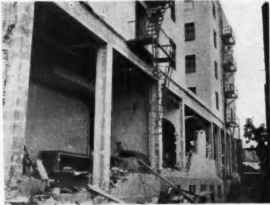
FIG. 5. SHOWING TYPICAL DESTRUCTION OF TERRA COTTA WALLS WITHOUT INJURY TO FRAME
